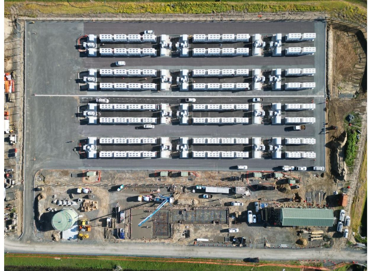
Completed container installation at Meridian's Ruakākā Battery Energy Storage system near Whangārei
