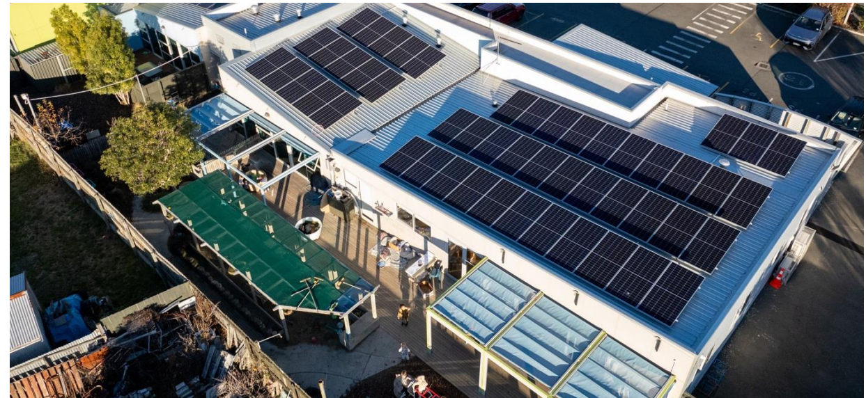
Solar installation at Waipuna Community Services in Canterbury
