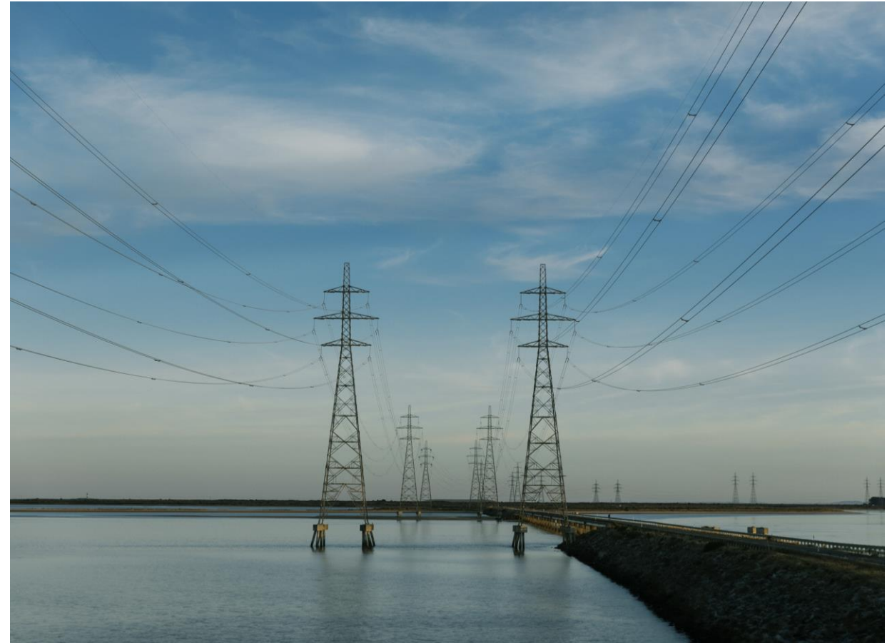
Transmission lines near New Zealand's Aluminium Smelter in Southland
