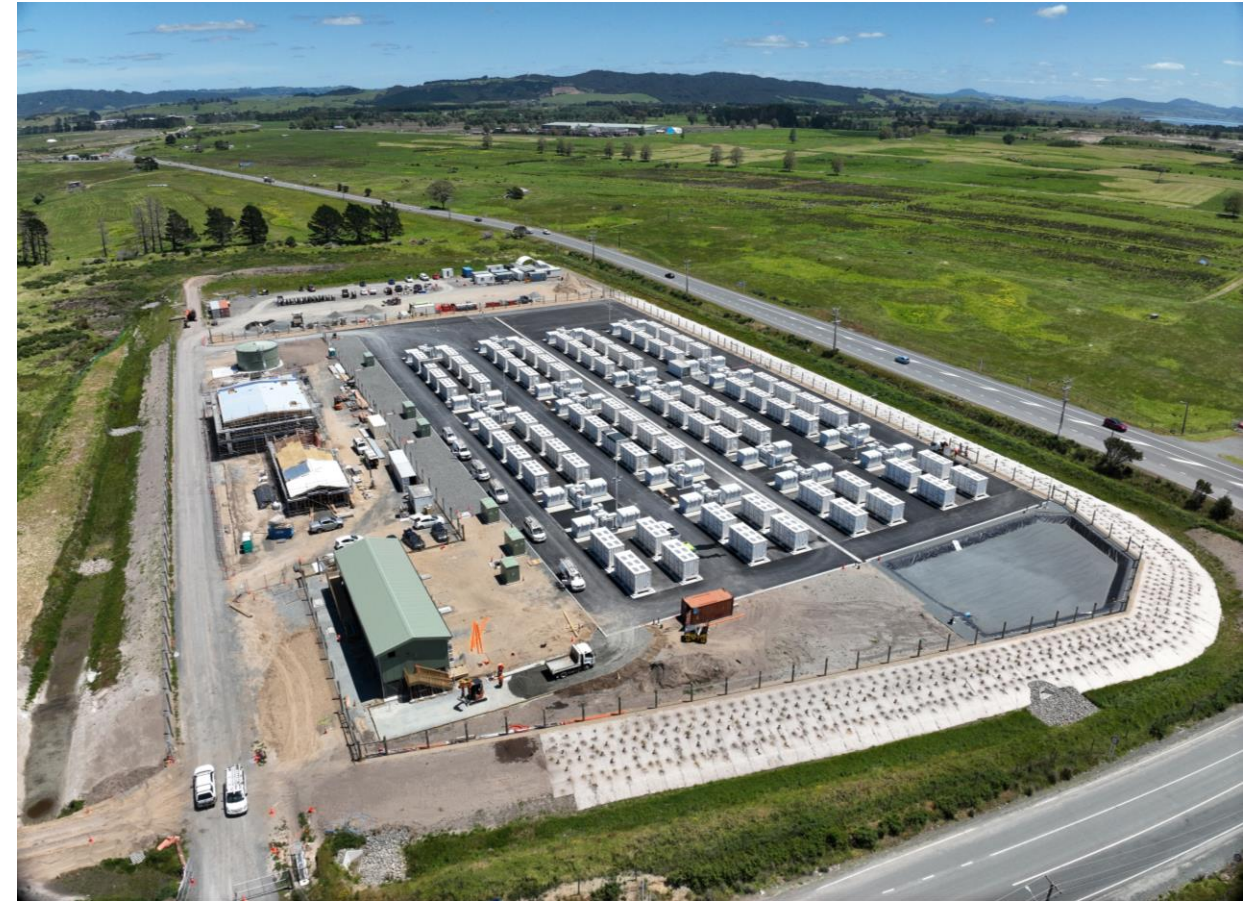
Meridian's Ruakākā Battery Energy Storage System near Whangārei
