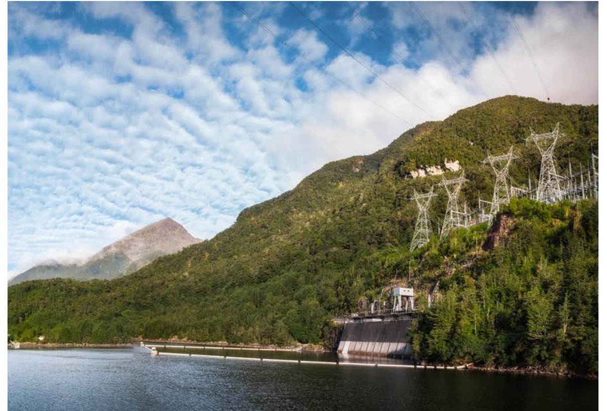
Meridian's Manapōuri Power Station in the Fiordland National Park
