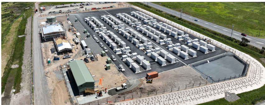
Ruakākā BESS development taken from a drone.
